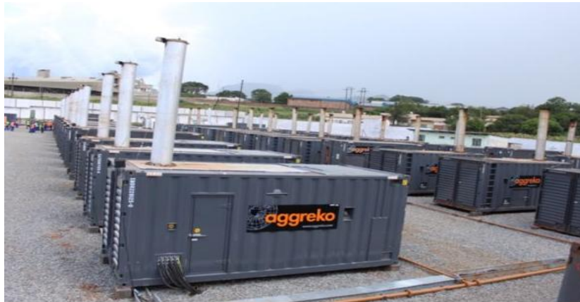
Fig. 7. Diesel generators in operation in Malawi
