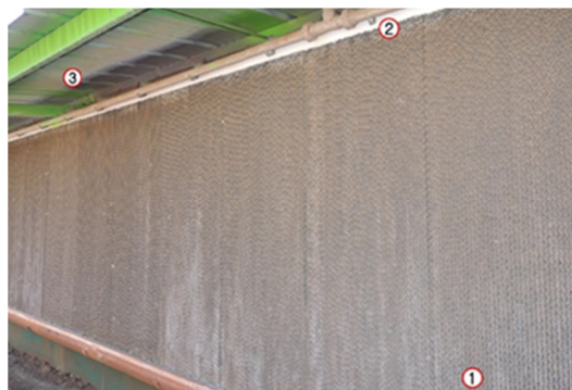
Figure 8. Cooling system—Pad cooling. Cellulose evaporative panels' side view. (1) Cellulose boards (2) Pad cooling hydraulic network system (3) Aluzinc tile trapeze TRP 35 with eaves with one meter
