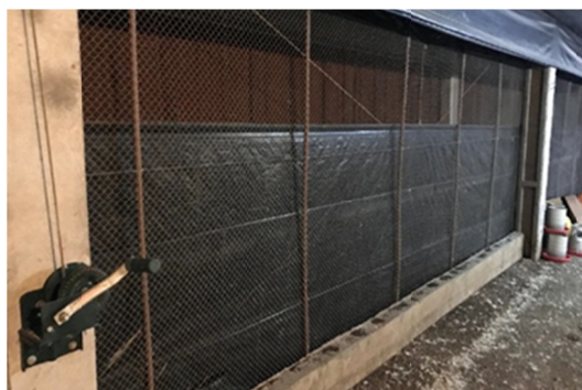
Figure 9. Cooling system—Pad cooling with manual air control
