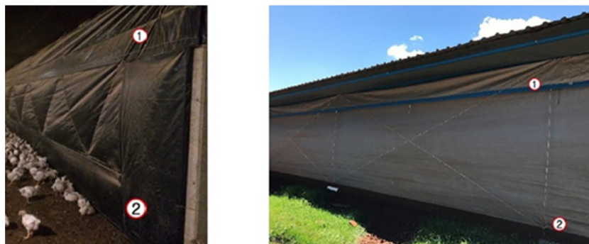
Figure 4. Side sealing of the poultry house A2. Detail of the side sealing. (1) Y type band with eaves internal face in black color and external face in silver color (2) Curtain internal face in black color and external face in silver color
