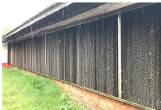
Figure 10. Cooling system—Pad cooling
