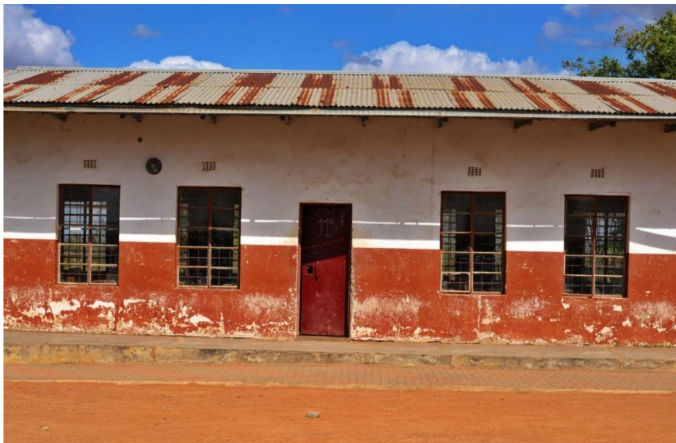
Fig. 2. Netshimbupfe Secondary School. (Example of schools still found in South Africa. However, there are number of new ones built but still having huge backlog in some areas. This is Netshimbupfe Secondary School block built in 1975.) Photo by Lucas Ledwaba, 8 June 2020
