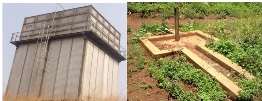
Fig. 5. Abandoned storage tank and stand tap
